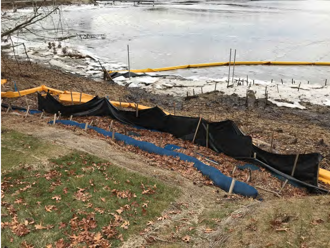
Fig 11: Toe of the slope at Gundalow Landing/east side of the bay. Viewing south. (01-26-21)
