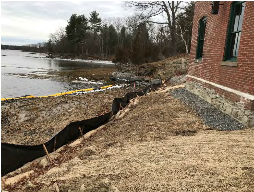
Fig 2: Slope between the cable house and salt marsh restoration at the Eversource property/west side of the bay. Viewing south. (01-26-21)
