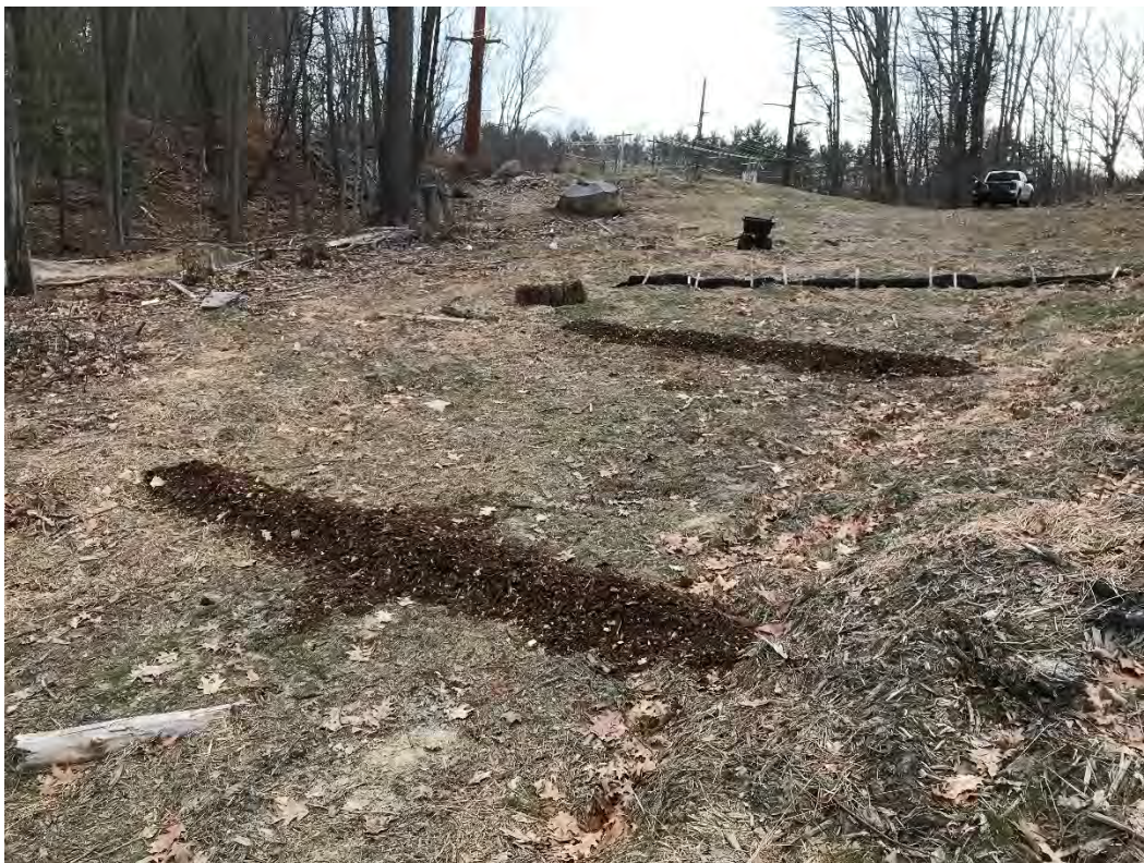
Fig 8: Upper portion of slope between Strs. 28 and 29. Viewing southeast. (01-26-21)
